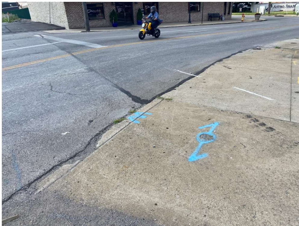
Figure 13 - Curb flush with the roadway at the inside of the curve, east side of South Bridge Street, north of the railroad.
