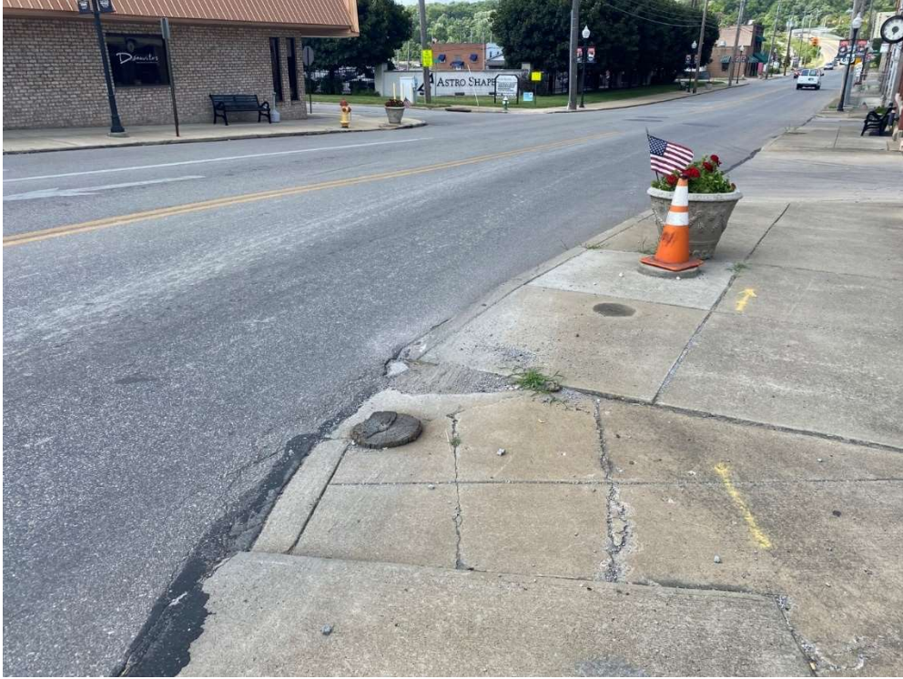
Figure 14 - Inside of curve, east side of South Bridge Street with cut-off pole and tire marks over the edge.
