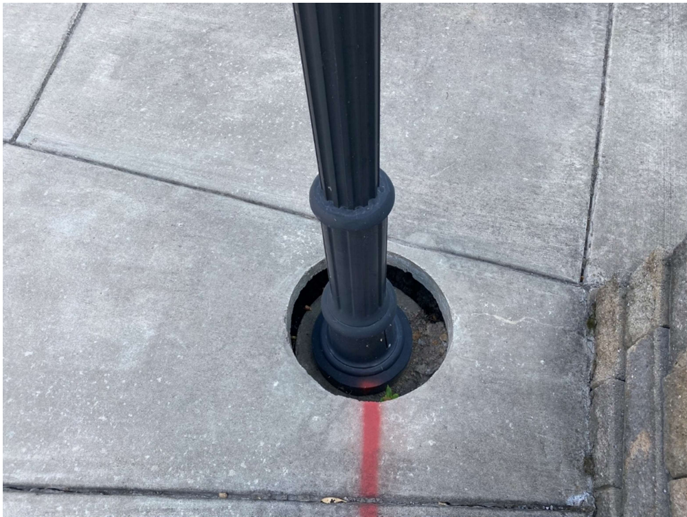
Figure 9 – Evident recent work with light poles.
