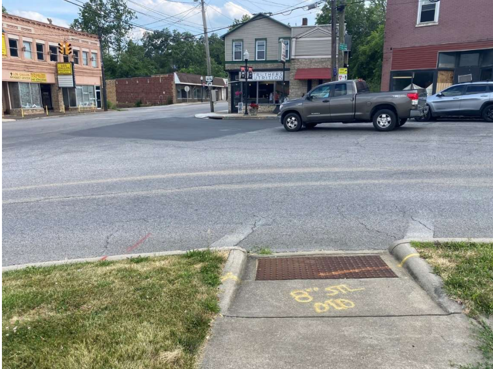
Figure 17 - Faded crosswalk markings.
